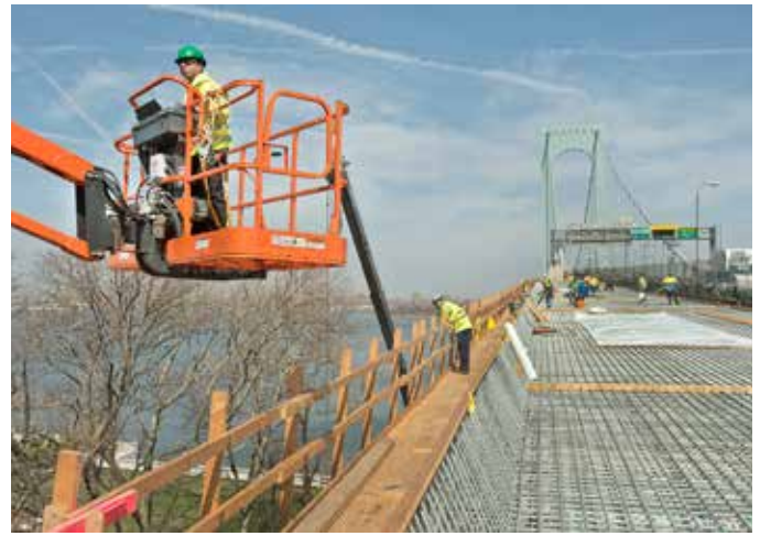
The Whitestone Bridge in New York is usually under construction. (NYC Metropolitan Transportation Authority).
